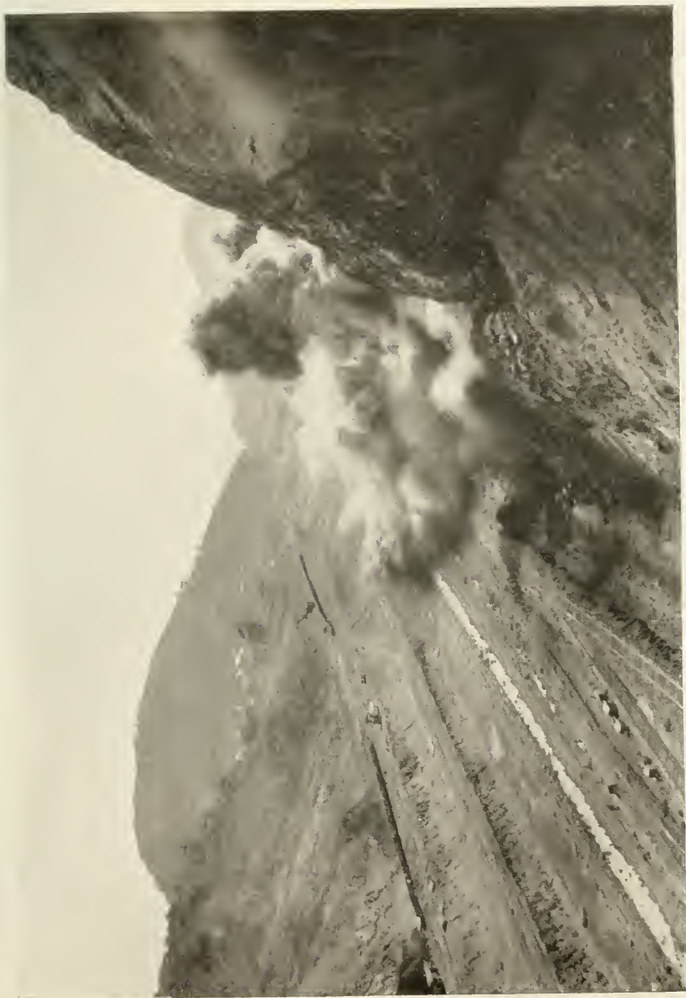
CULEBRA CUT AT CULEBRA: VIEW LOOKING SOUTH; BLASTING ROCK ON CONTRACTORS' HILL, JANUARY, 1912.
